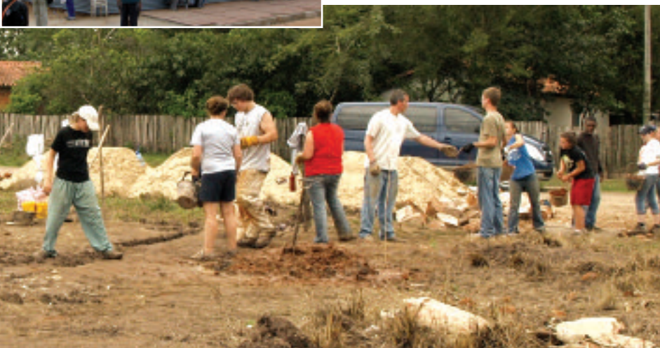
Bottom photo: During the group's Habitat for Humanity service project near Mennonite World Conference, some of the workers formed a "bucket brigade" to supply the other workers with construction materials they needed for the foundation of the home they helped to build. PHOTO: PETER BRUBAKER
