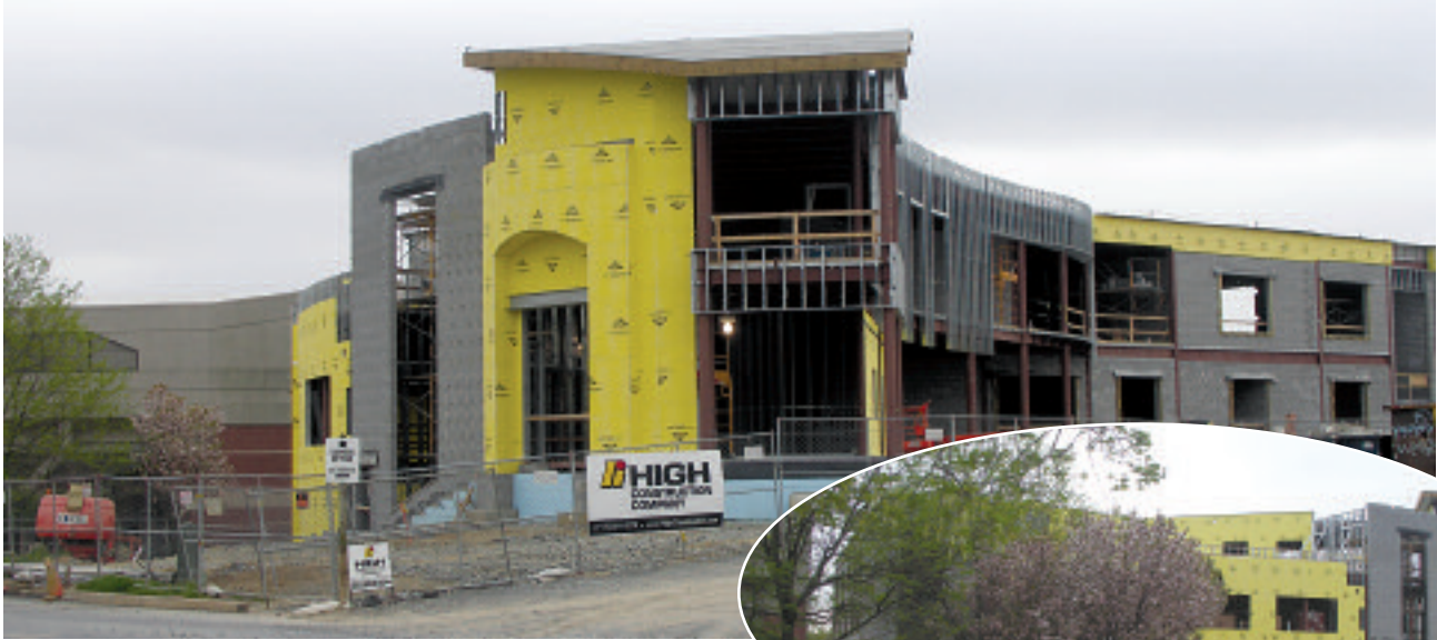
The academic building taking shape at the Lancaster Campus is set for an autumn completion. The facility will include classrooms for math, science, business, and family and consumer science, along with offices for system personnel.
